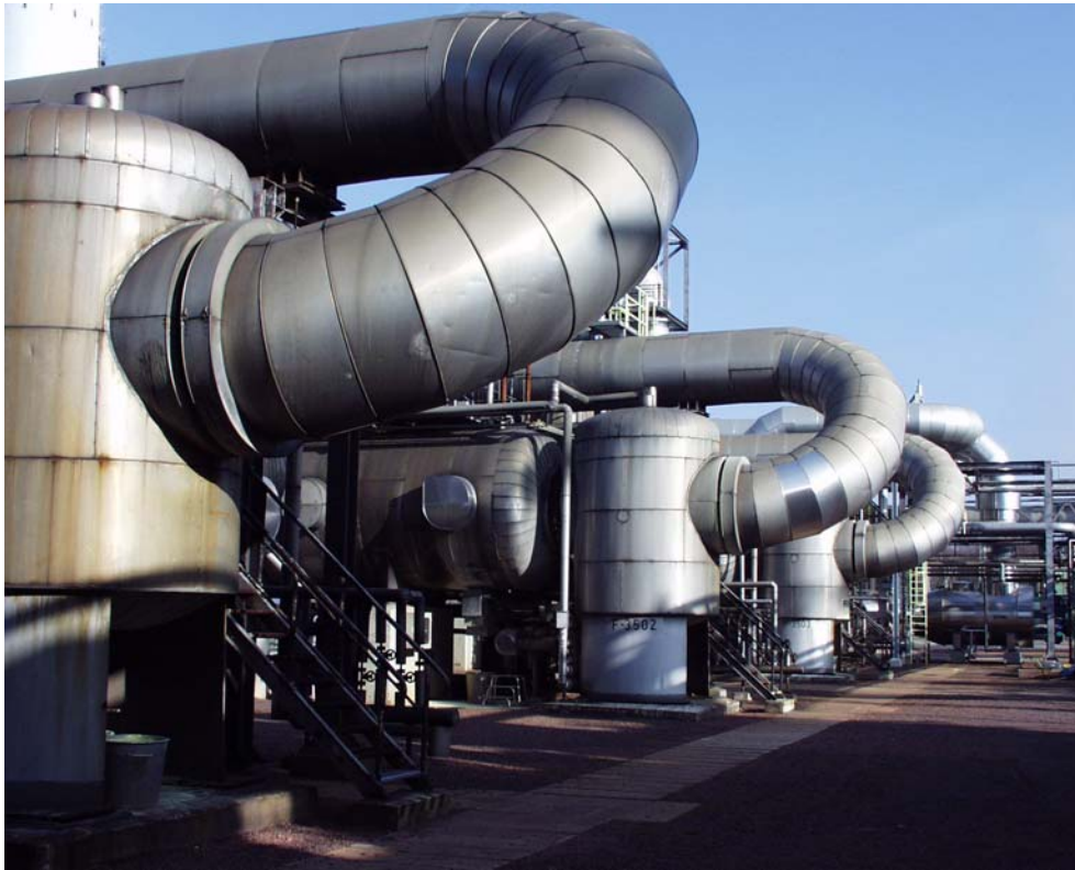
Figure 3: A 700 t/d Claus plant at NEAG Voigtei, Germany
